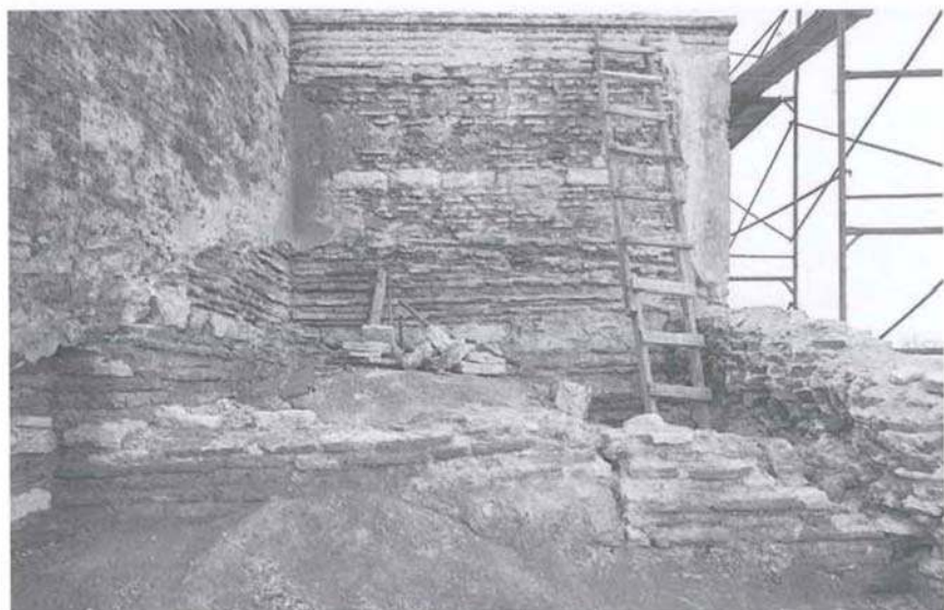
Figure 2. Zeyrek Camii, north church, roof of north-east corner, with the partition wall in the foreground (Z. Ahunbay, 1998).
